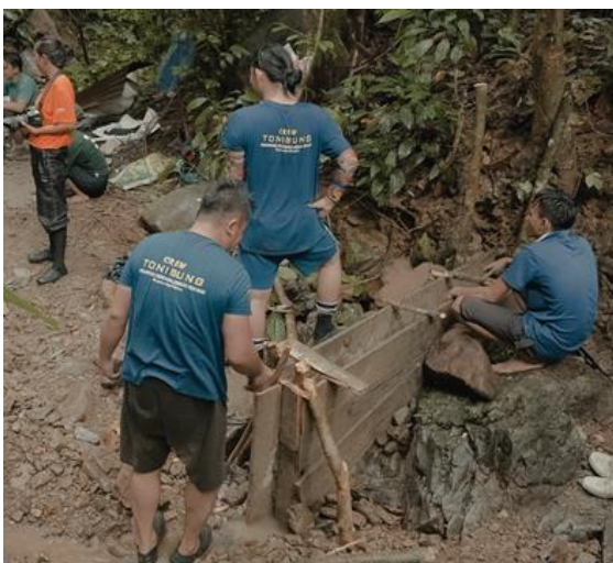
Left Photo: Micro-hydro Installation Site © Forever Sabah
